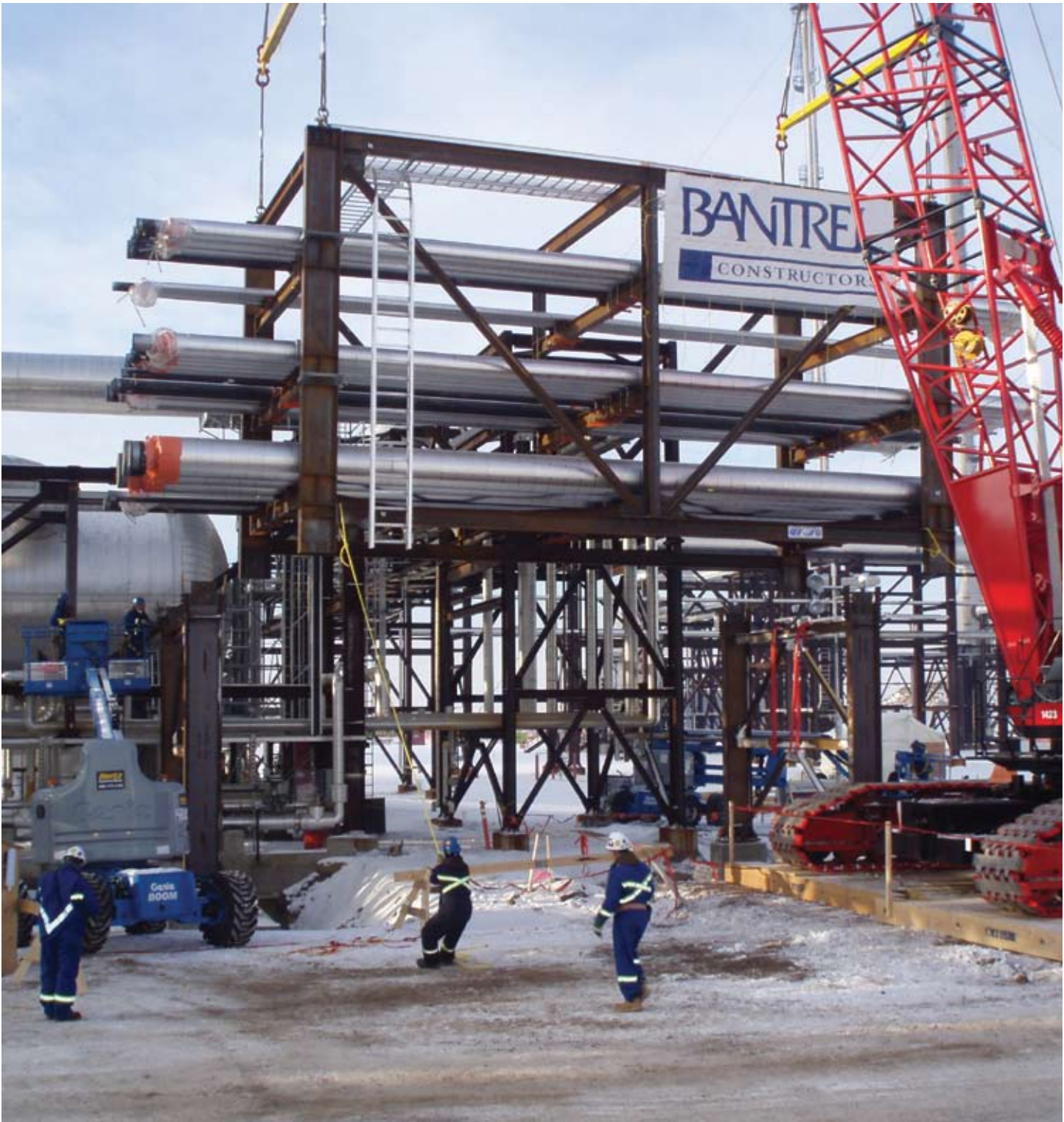
The Bantrel Constructors' flag flies proudly at the Scotford Upgrader Expansion site.
