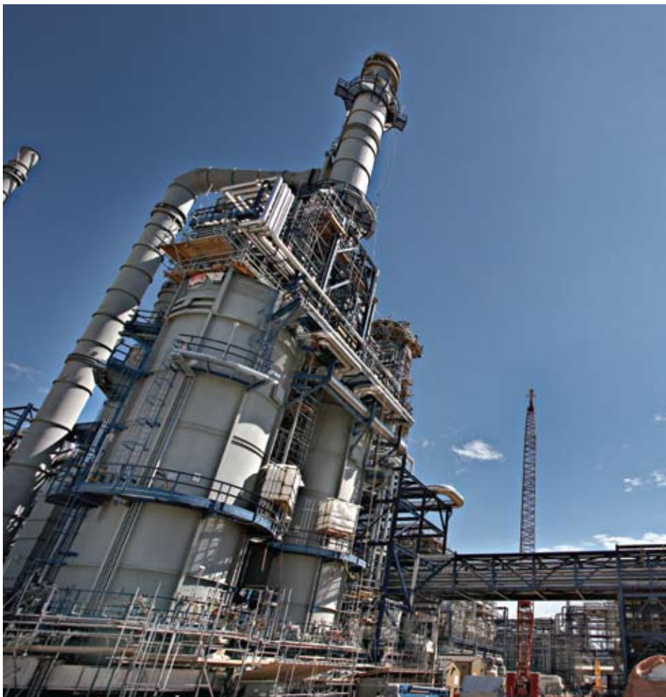
The Crude Heater on the Crude Vacuum Unit at the Petro-Canada Refinery Conversion Project in 2008.
