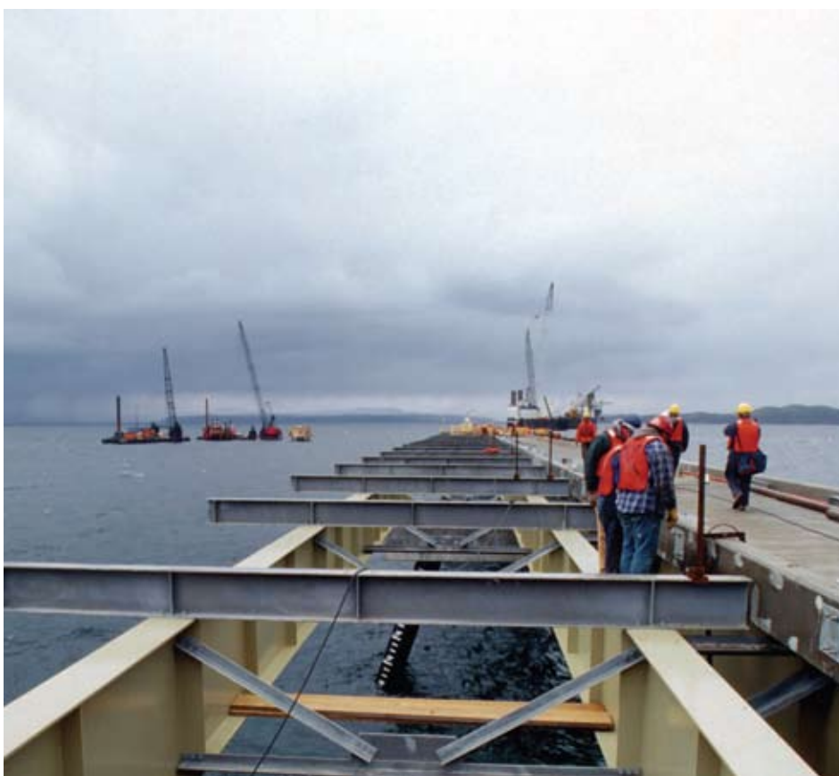
Bantrel field engineers are shown in this 1997 photo overseeing construction of the terminal.
