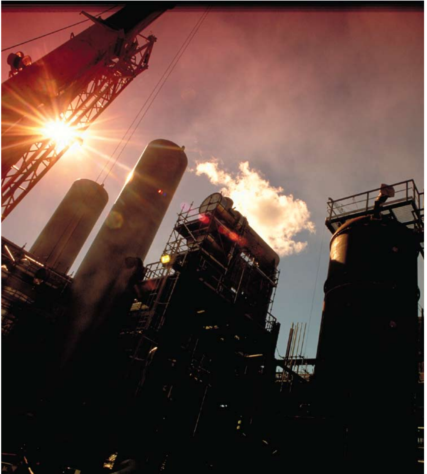
A view of the Millennium coker structure at dusk.
